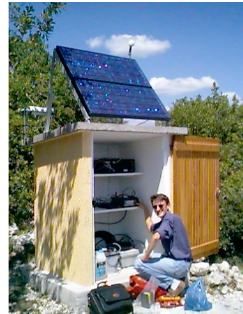
Shelter with GPS receiver, solar panels
